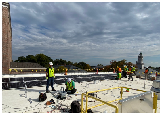
Sixty solar panels make up the Curtis Media Center’s 25.2 kW system.
